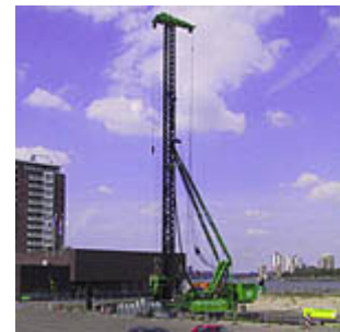
Construction began with dam walls being pile-driven to a clay layer 107 feet (32.5 meters) deep. Photo: Architectenbureau de Ruiter b.v.
